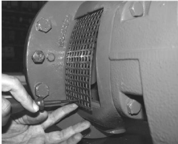
Figure 7: Motor lantern screen removal
